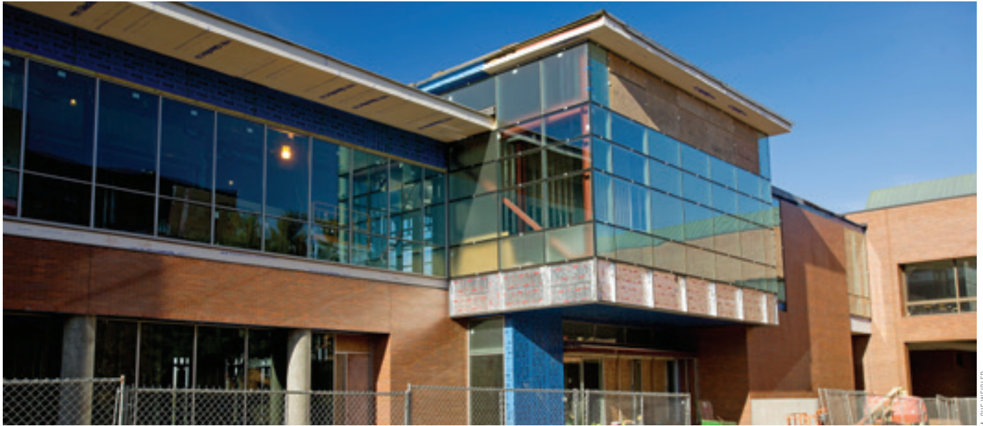
Creating an Innovative Space Construction continues on Sebastian and Lenore Rosica Hall, slated to open in October.
